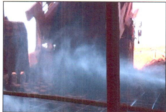
Photo 11 : Showing Operation of Dry fog system in Crusher
