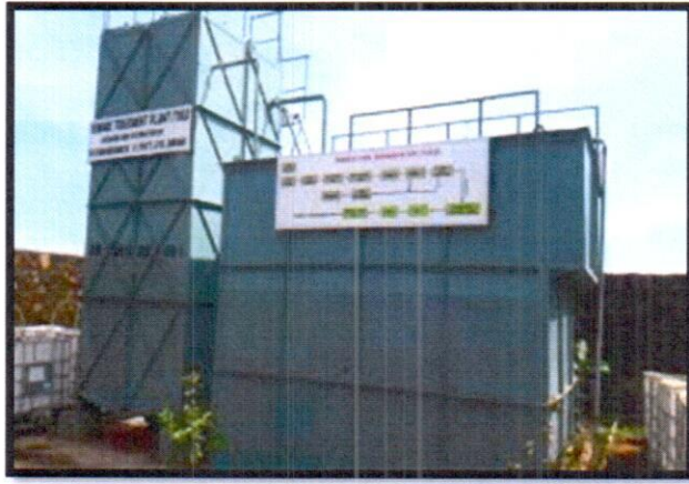
Photo 12 : Showing Sewage Treatment plant for Treatment of Domestic Waste Water
